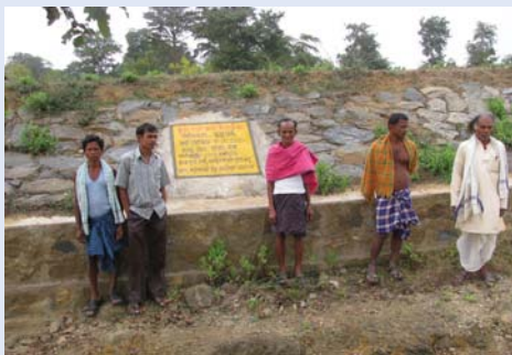
User Group members benefitting from Guard wall against heavy run-off in Ainlabhat, Gaisilat, Bargarh
