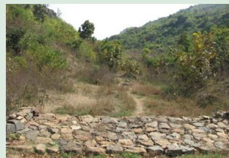
Loose Boulder Check Dam protecting land from run-off in Podapali, Khariar, Nuapada
